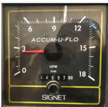
Photo 1: Flow meter readout display in tank building.
